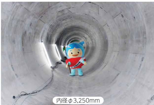
【大石2号貯留管】貯留量16,700m 3
